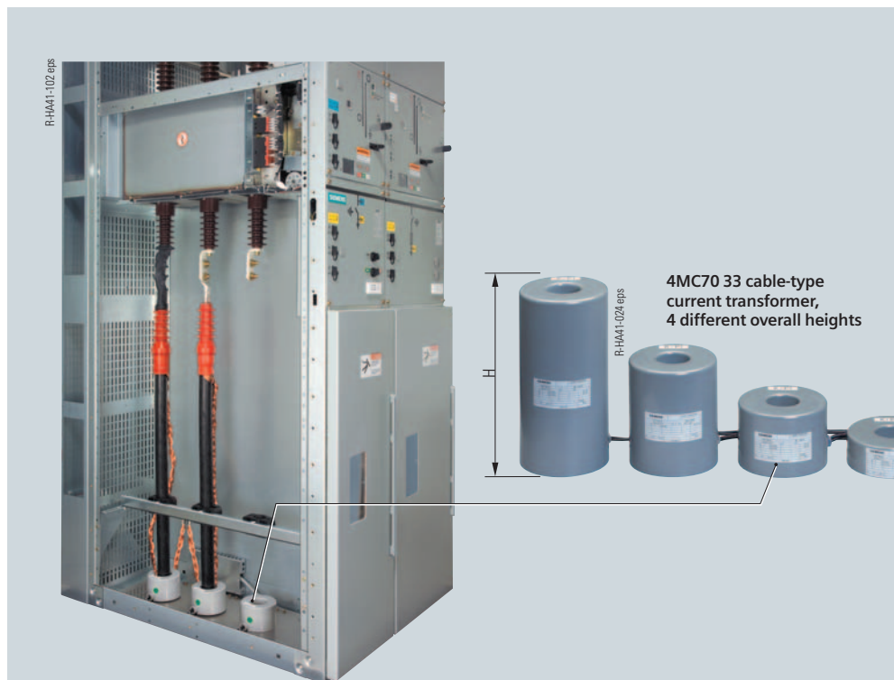
4MC70 33 cable-type current transformers on the cable at the panel connection **
