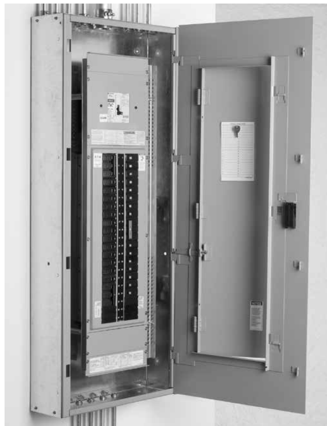
Trim Hanging on Surface Mounted Box
